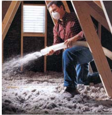
Blowers make the job easier and are available at most home centers selling blown insulation. You will need help loading the hopper with material or you will have to make several trips up and down the ladder.
