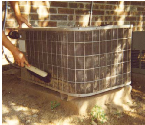
Keeping the outdoor compressor free of dirt grass and other obstructions is important to reduce operating cost and prevent equipment failure.
