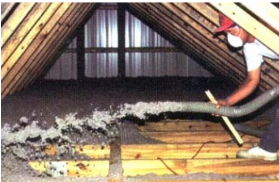
Attic insulation slows heat loss in the winter and stops heat gain in the summer. Insulation and proper attic ventilation are important for comfort and efficiency.
